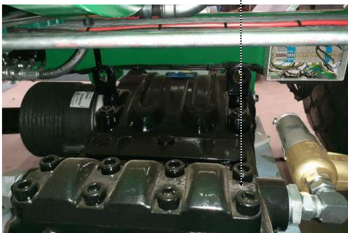
Spulepumpe placeret under tanken
